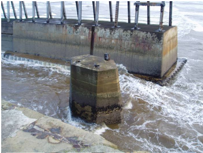
Figure 21 West Face of Pier extension with subsided pillar in foreground
